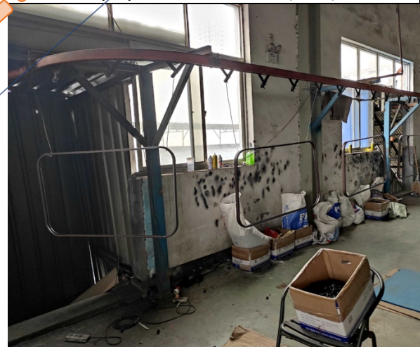
Equipment-Powder coating line-1set
