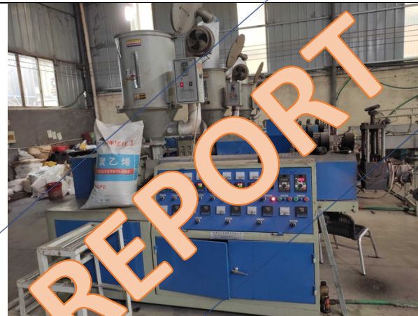
Equipment-Injection line – 3 sets
